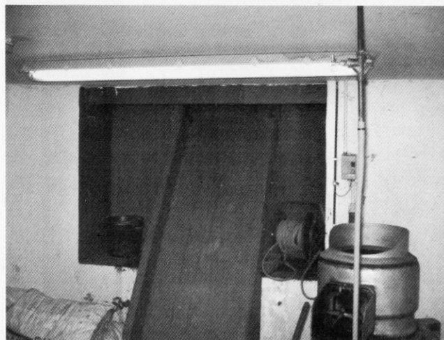
The basement of the Sandgrounder chippy showing one of the original windows that that has now been blocked up. Photo by Andrew Smith
